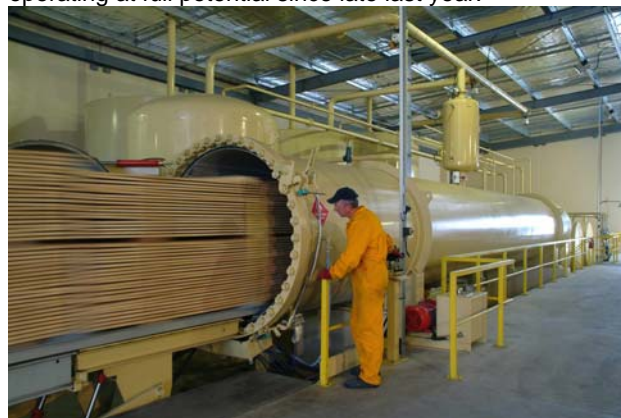
The new LOSP plant in operation.
